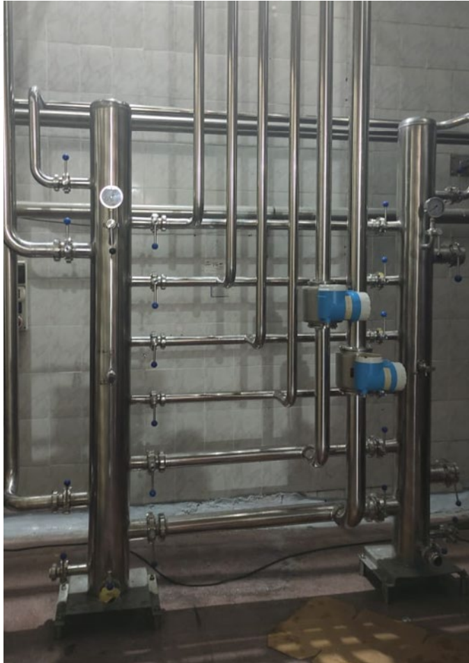
Treated water distribution Manifold S.S 316 L
